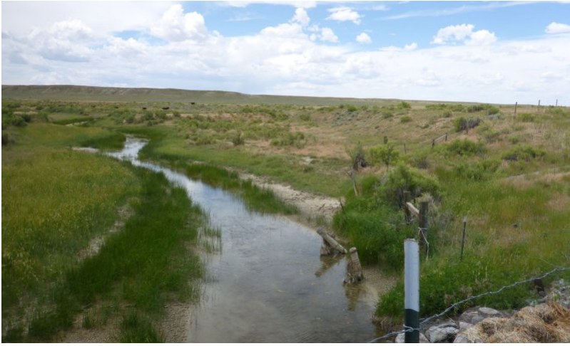
Figure 15. Evidence of the old road bed in the upper portion of the photo and the current road bed with the remnants of an old head gate are a few of the disturbances to this site.
