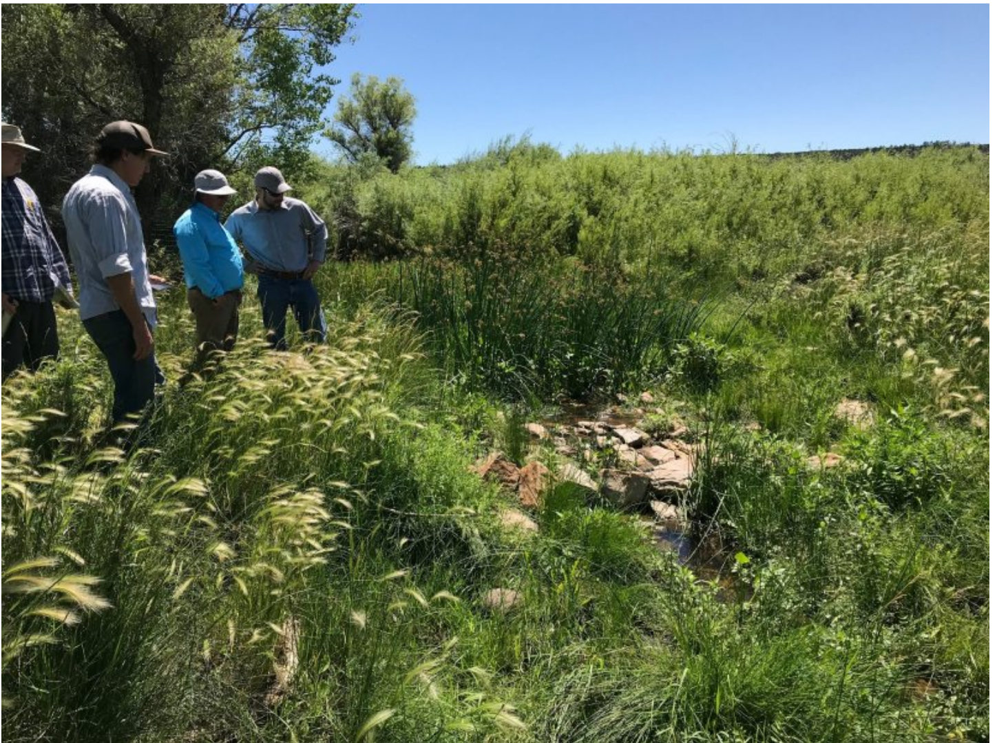
Figure 7. Riparian restoration along a section of formerly incised channel in the form of grade control structures such as 1-rock dams. Intended to reconnect parts of the floodplain to the water table.
