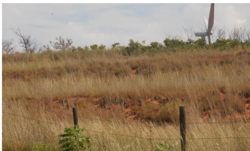
Figure 25. Eroded Quinlan soils. Community 4.1 Dewey County, OK
